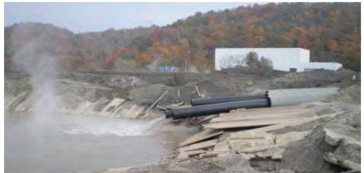
Pipes entering a coal ash pit at the J.M. Stuart Station, located in an Ohio River flood zone.
